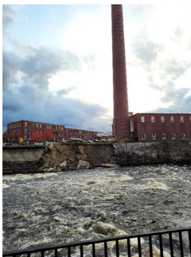
Photo 1 A section of the stone riprap along the Saco River in the Biddeford Mill District was damaged during an extreme precipitation event and subsequent high River flows in late October 2021. Credit: A. Sherwin
